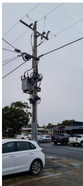
Figure 10 Venus Bay Shops and transformer
